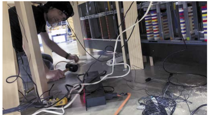
Blake Foster works on the growing mass of wires under the table of New Hashima. Photo By Simon Liu.
